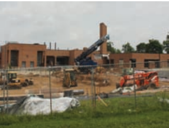
Renovation and expansion of the Livestock Disease Diagnostic Center is under way. This photo was taken in July 2009.
