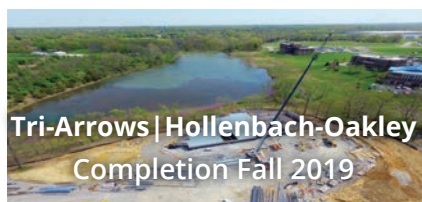
Quadrant Magnetics Completed 2019
